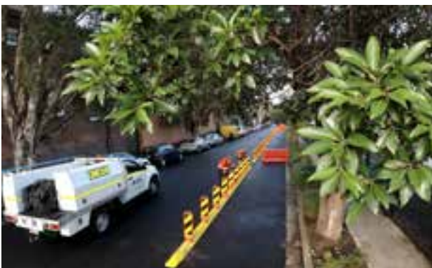
Figure 6.3 Installing the infrastructure required to support a pop-up cycleway is relatively quick and simple, as demonstrated on Henderson Road (Credit: Transport for NSW)
