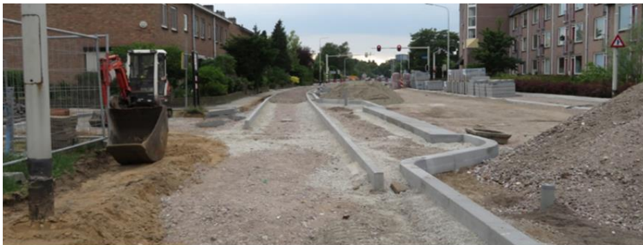
Figure 4.3.1(B) – Retrofitted protected unsignalised intersection with 2m buffer and flush kerb running both sides of the cycle track, part way through construction and finished, Nijmegen.
